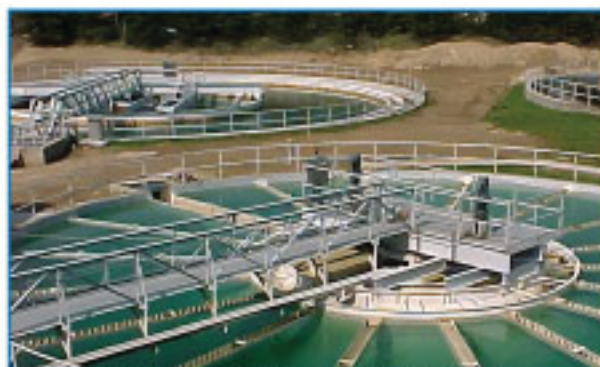
WTP & STP Treatment Plants
